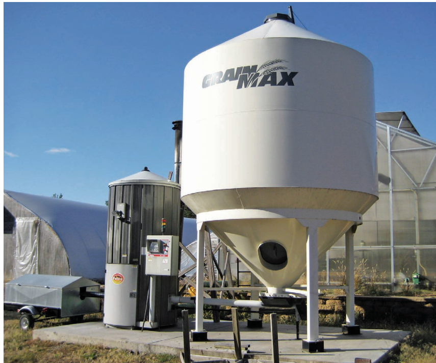
Hydronic pellet boiler with pellet storage bin.
