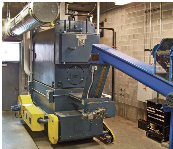
Hydronic pellet boiler with pellet storage bin.
